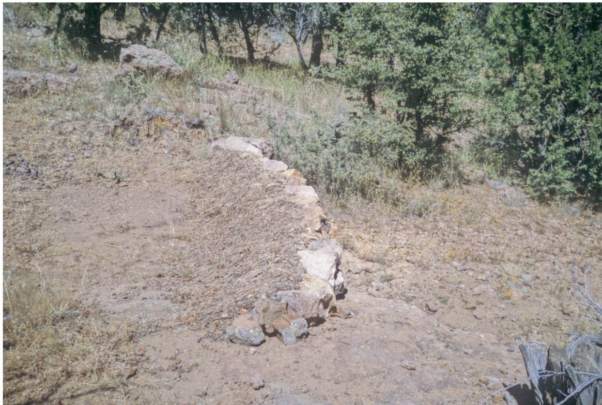
Figure 2. Loose rock dam on Joe Austin ranch 1993. Note debris on upside of dam indicating that it ran over.
